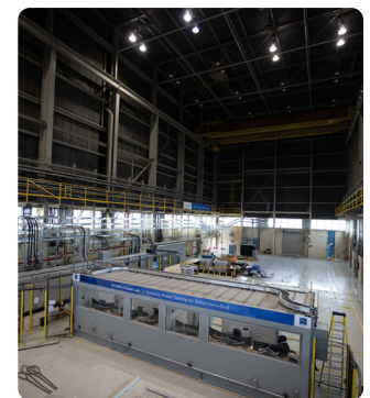
GridSim Power Lab
