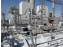
In-situ transformer testing
