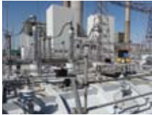
In-situ transformer testing
