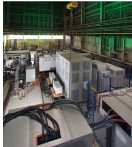
GRIDSIM Power Lab
