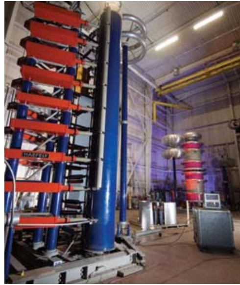
High Voltage Lab
