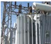
Distribution station equipment
