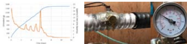
Figure 2. (Left) Leak / time chart for ANAGEN™ in open air showing complete leak cessation. (Right) Image following test completion showing build-up of cured material on leak site. Cable pressure constant at 30 PSI.
